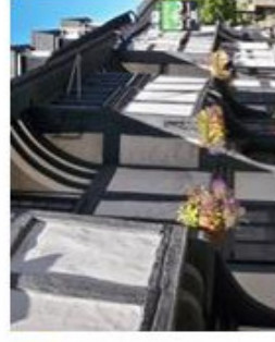
Wealden houses have curved straps that support the hall roof. There are two in Weobley.
